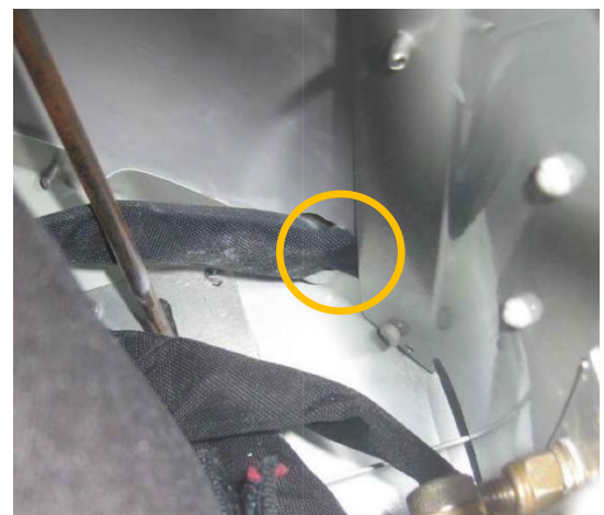
Fig. 3: picture taken from an installation Inside showing the hole in the egress panel
